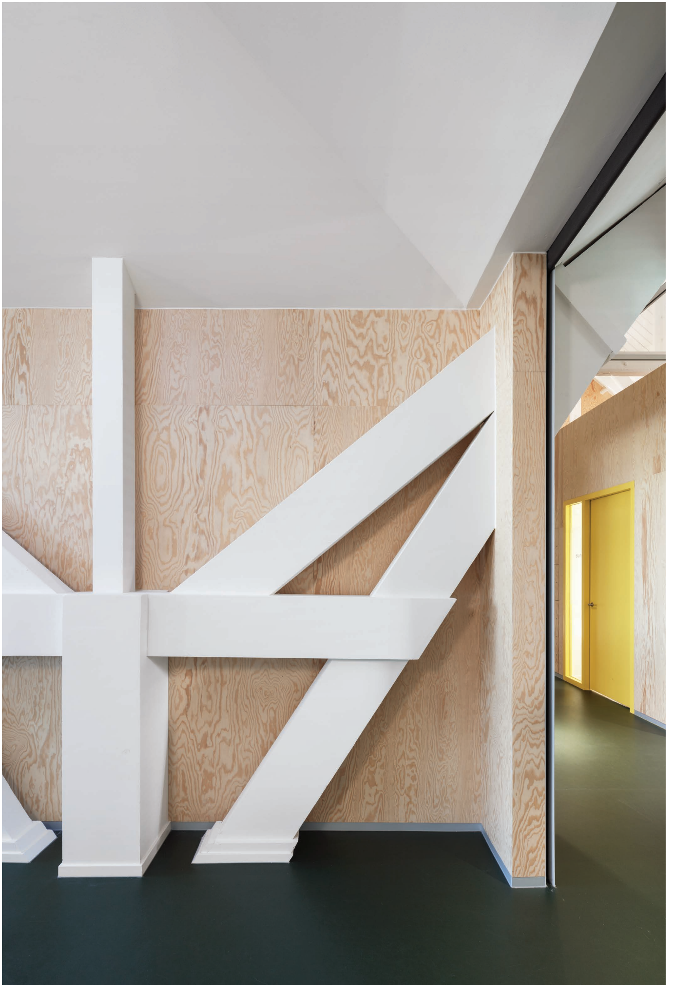
The characteristic construction of the gable roof is visible in the 'new' office landscape.
